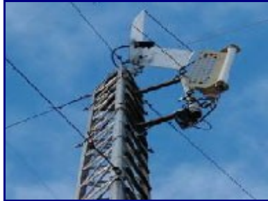
Figure 2: Solectek Antenna installed in Mérida, Venezuela, 1997 as part of RETIEM, (Merida State Teleinformatic Network) with links of up to 40 km.
