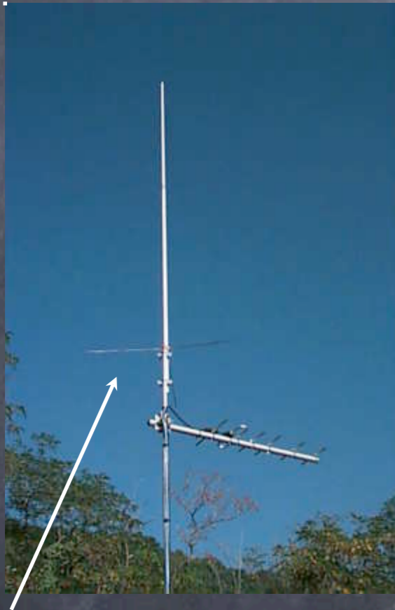
Omni Directional Antenna
